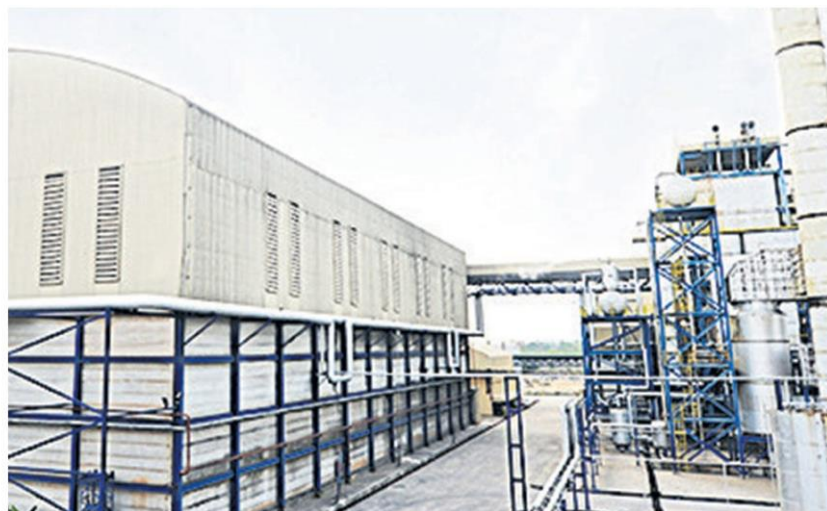
Buriram Sugar's biomass power plant in Buri Ram, which hopes to win a PPA.
